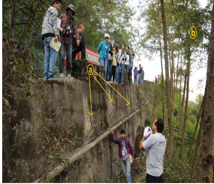
Figure 2.8: (a) Rock anchoring structure at Khawa, Dhulikhel, in the Araniko Highway, central Nepal, for protecting the road by stabilizing the slope. (b) Bio-engineering system utilized to control the slope (Photo: Field excursion during the symposium, MGDA-11).
