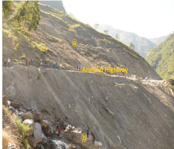
Figure 2.9: (a) Large scale landslide width of the 755 m on the north of Bahrabise and located on the left bank of Sunkoshi River along the Araniko Highway, central Nepal. (b) Gabion is being constructed to stabilize the slope to protect the part of Araniko Highway from further landslides (Photo: Field excursion during the symposium, MGDA-11).
